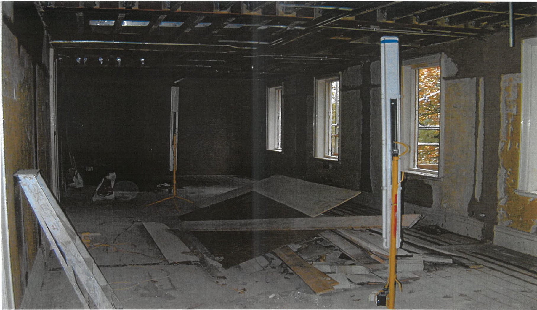
THE NEW DISASTER RECOVERY ROOM (APT NAME LOOKING AT THE PICTURE) THREE INTERMEDIATE WALLS HAVE BEEN REMOVED TO CREATE THIS SPACE. CLOSE EXAMINATION OF THE PICTURE SHOWS THE NEW STEEL JOIST AT CEILING HEIGHT.
