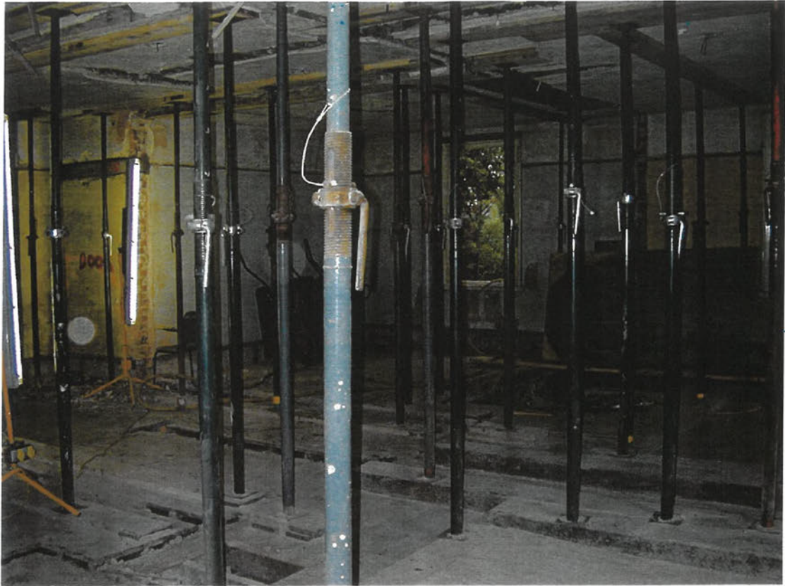
NEW GROUND FLOOR TRAINING AREA
