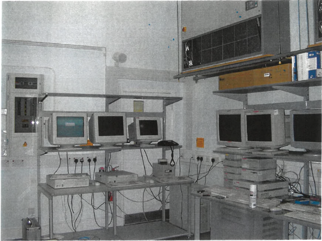
NEW IT BACK-UP SERVER ROOM
