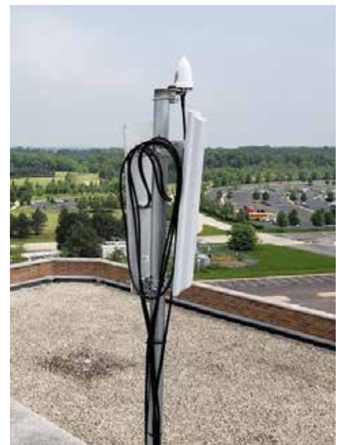
CBRS 3.5 GHz MIMO equipment installed by ExteNet.
